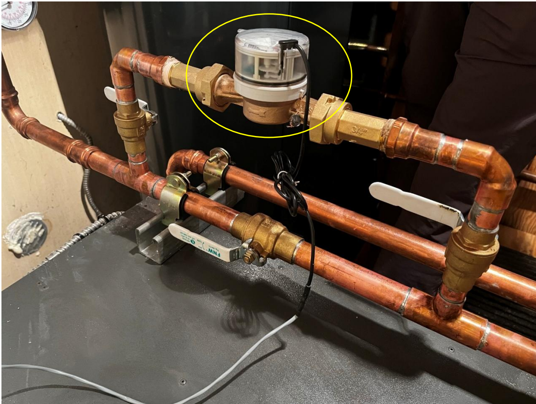
Figure 2.6 – In-line flow meter installed to measure the volumetric flow rate of the glycol solution being delivered to the heating/cooling loops in the home by an air-to-water heat pump.
