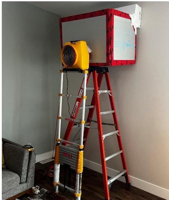
Figure 2.5 – Apparatus used for measuring the in-field flow rate (CFM) of indoor heads using a rigid airtight plenum, flow-adjustable fan, and manometer.
