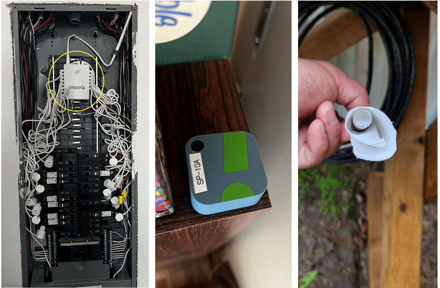
Figure 2.7 – Sub-metering equipment in electrical panel for measuring supplemental electric heating (left), sensor for measuring ambient indoor air temperature and relative humidity (middle), and sensor for measuring ambient outdoor air temperature and relative humidity (right).
