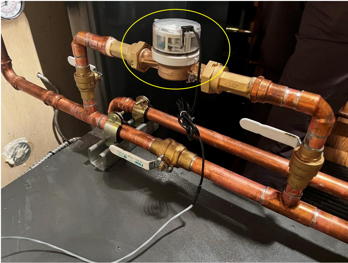
Figure 2.6 – In-line flow meter installed to measure the volumetric flow rate of the glycol solution being delivered to the heating/cooling loops in the home by an air-to-water heat pump.
