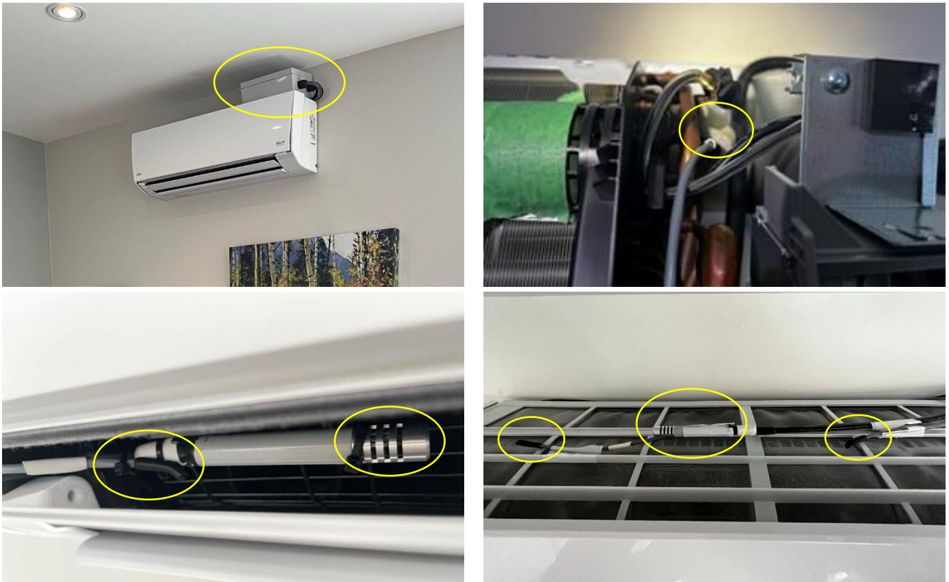
Figure 2.3 – Mini-split indoor head with monitoring equipment box (top left), surface temperature sensor at the vapour line (top right), and temperature and relative humidity sensors at the supply louver (bottom left) and at the return louver (bottom right).
